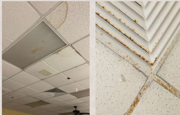
Moisture damage causing rust and damage
